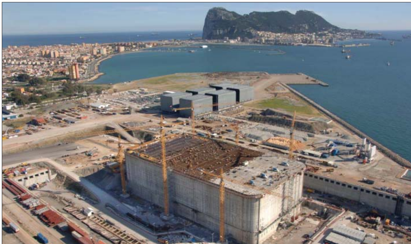
Construction of the tanks for Italy's Adriatic LNG terminal progresses in Algeciras, Spain. Capable of storing 250,000 cu m of LNG, the tanks were floated out in November 2006 to the terminal's site in the Adriatic Sea about 15 km off the Levante Po River. Photo from Adriatic LNG.
