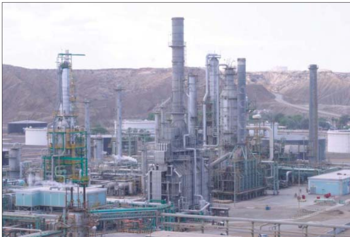
Planned construction of Petroperu's Talara refinery includes several new processing units as well as expanded crude and vacuum distillation units. Project completion is due in January 2012. Photo from Petroperu.
